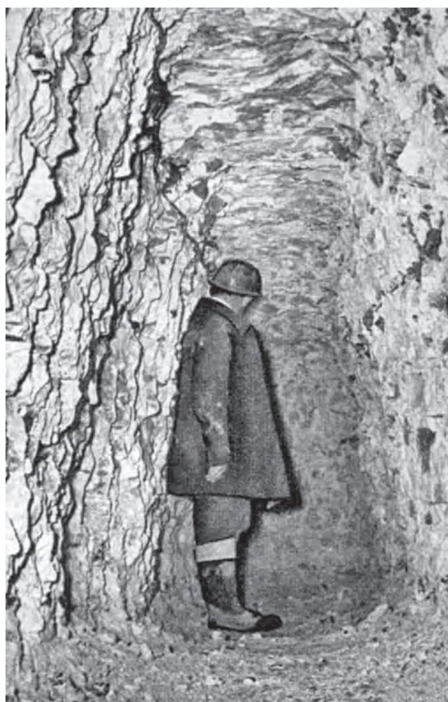
Sixty feet below Plumstead garage Charles Marshall of the Chief Civil Engineer's department inspects a tunnel in the chalk
